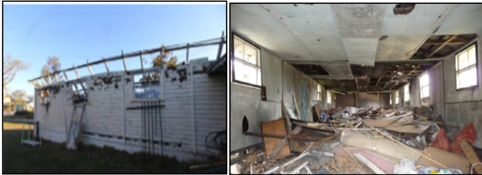
Figure 29 – Current condition of the Army Mess and Kitchen. Source: Figure 169 and 170 of the draft CMP.
